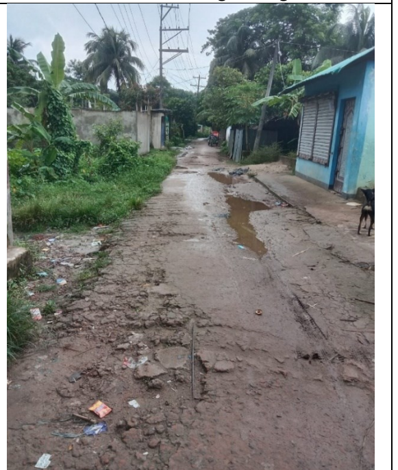
Photo SP.RD8.001: Existing Damaged RCC Road
