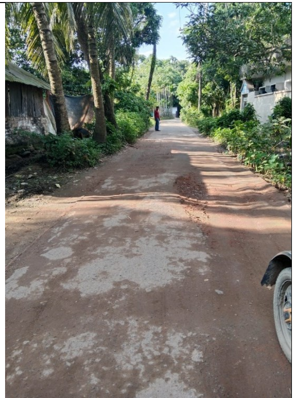
Photo SP.RD2.001: Existing Damaged BC Road
