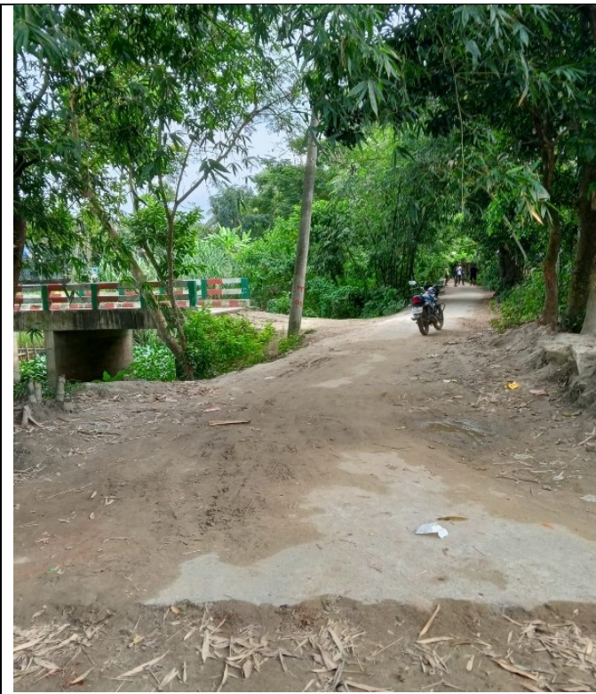
Photo SP.RD1/4/5.001: Existing Damaged BC Road
