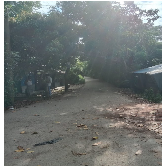
Photo SP.RD2.002: Existing Damaged BC Road
